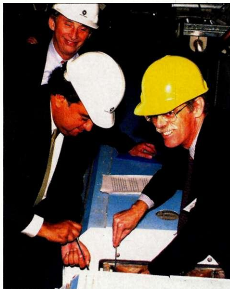
US Energy Secretary Bill Richardson helps install the final magnet in Fermilab's Main Injector Ring. Making sure all is well is Fermilab Director John Peoples (behind) and Main Injector Project Manager Steve Holmes (right).
